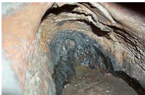
Rust \frac{3}{4} way through 6" steel cap
